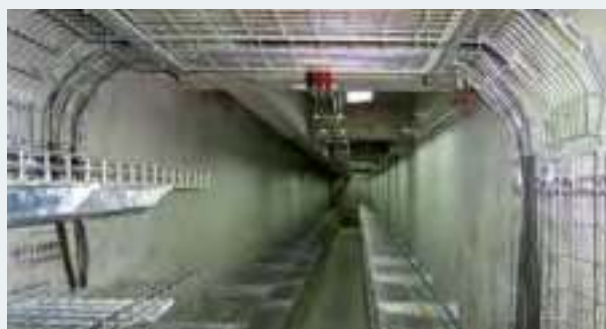
• Data Center Telmex / Regional Bogotá
