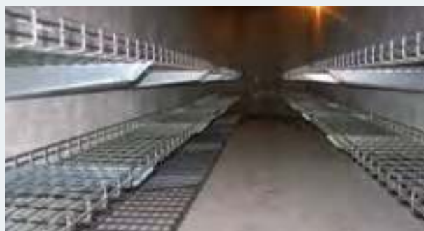
• Data Center Telmex / Regional Bogotá
