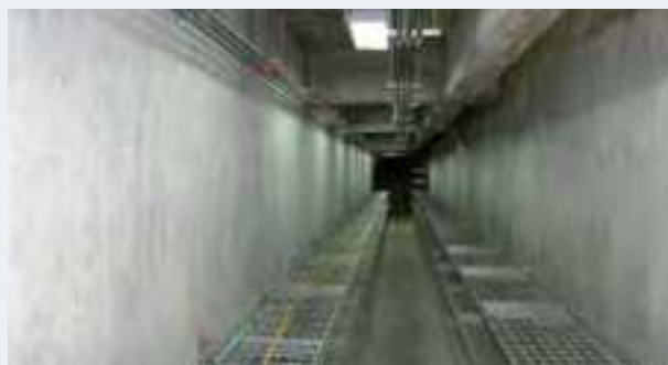
• Data Center Telmex / Regional Bogotá
